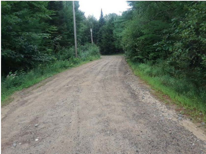
Rutting - Lord Road
