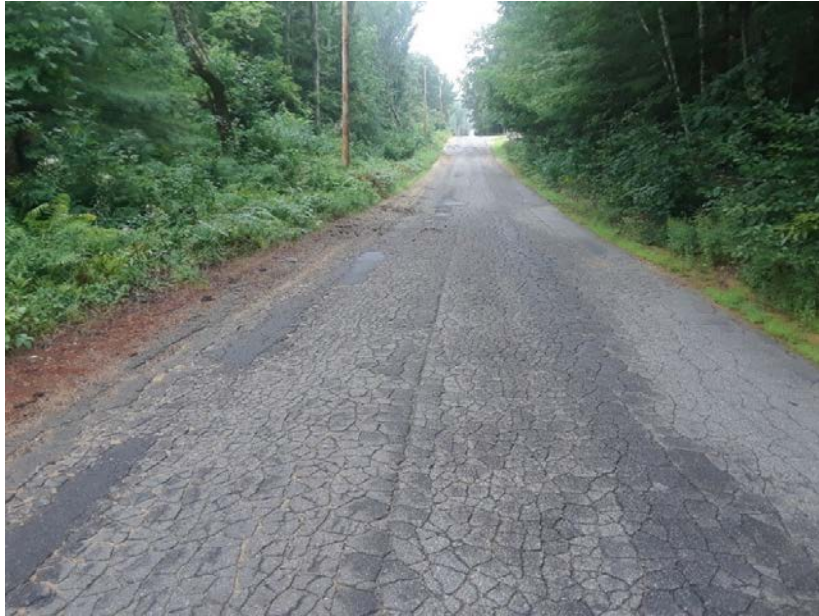
Alligator Cracking - Blanchard Road
