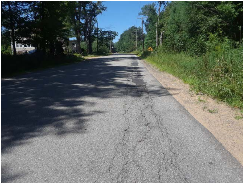
Rutting - Center Road
