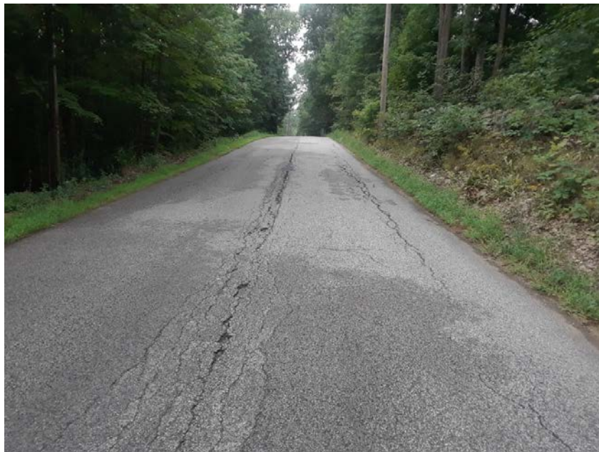
Longitudinal Cracking - Smith road
