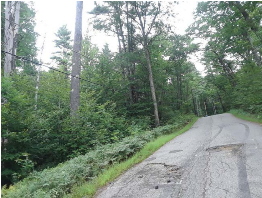
Patching/Potholes - Sewell Shores Road
