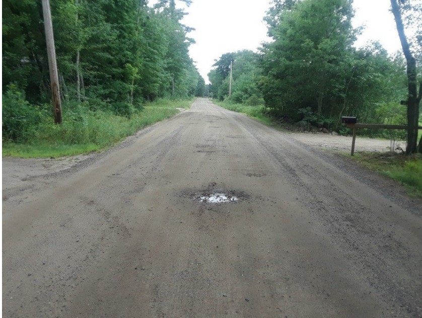
Potholes - Lower Guinea Road
