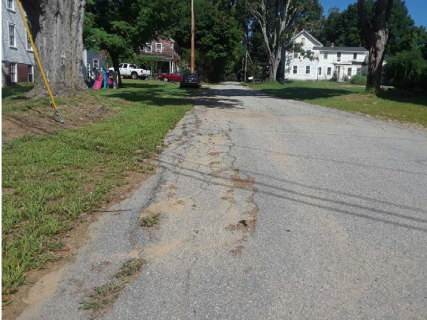
Edge Cracking - Academy Road
