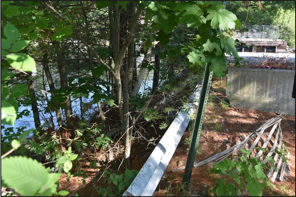
Figure 18. Steep fill slope along the western road edge near the bridge, view northwest.
